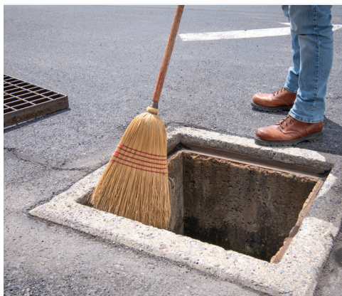
1. Remove drain grate and clean any sediment or debris from grate lip and ground surface.
